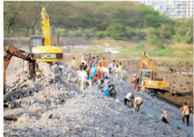
Fig. 3: Dumping of C&D waste illegally done at Pune City
