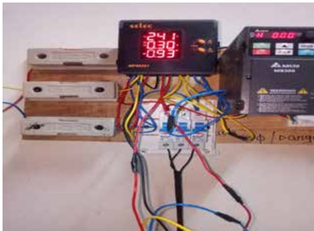
Fig. 4 Phase to neutral voltage, Phase current and PF without reactive load situation
