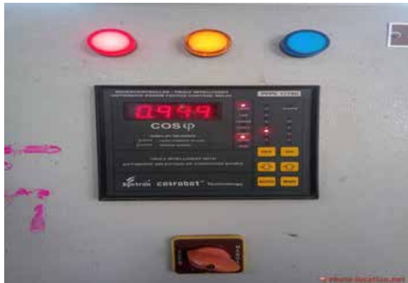
Fig. 8 APFC unit indicating unity PF
