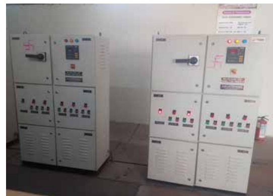
Fig. 7 30kVAR PFC unit installed with standby
